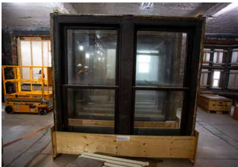
Old windows from Centre Block are lined up for removal on the fifth floor on Feb. 7. The Hill Times photograph by Andrew Meade
