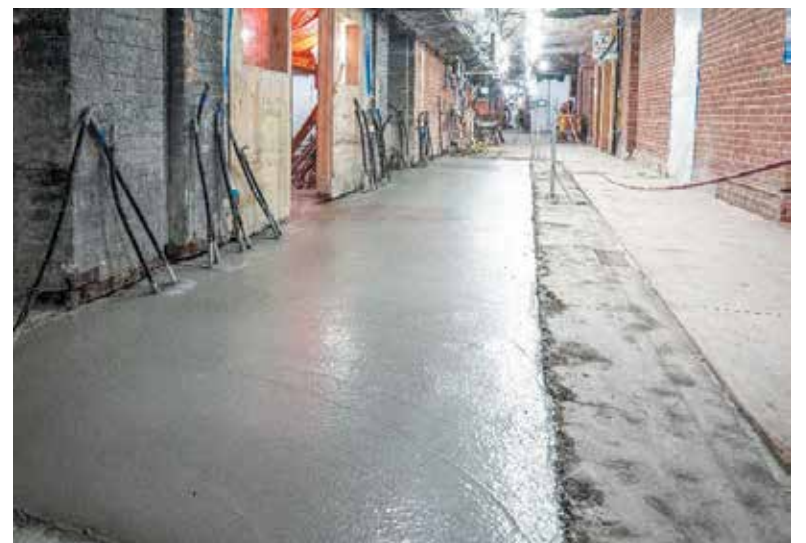
Freshly poured concrete as part of slab replacement work in the southwest corridor of the first floor of Centre Block. Photograph courtesy of PSPC
